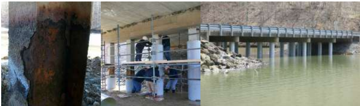
Figure 12. Rehabilitation of corroded steel H-pile bridge using composites, East Lynn Lake Bridge, East Lynn, WV. The repair cost 35% of the cost of a conventional repair. (WVU, 2014)
